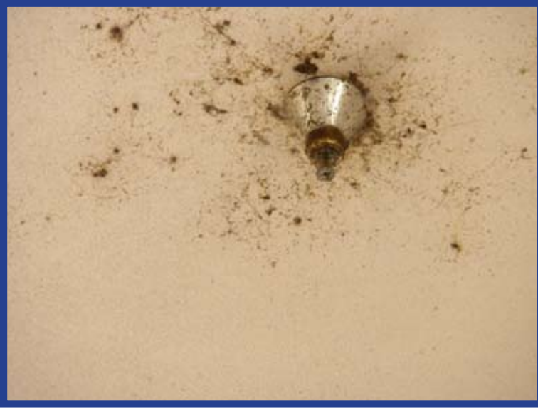
BEFORE: Sprinkler Thermostate Heads (not Protected)
