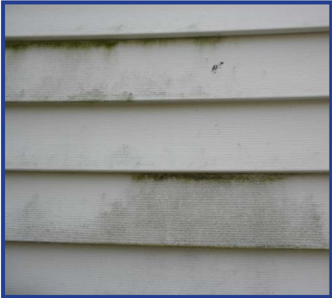
GREASE FROM GRILL-BEFORE
