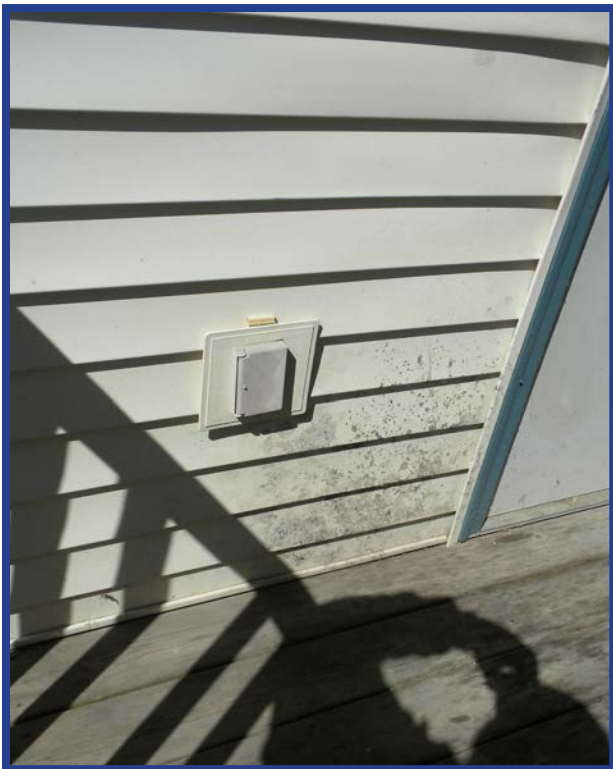
DECK & SIDING BEFORE CLEANING
