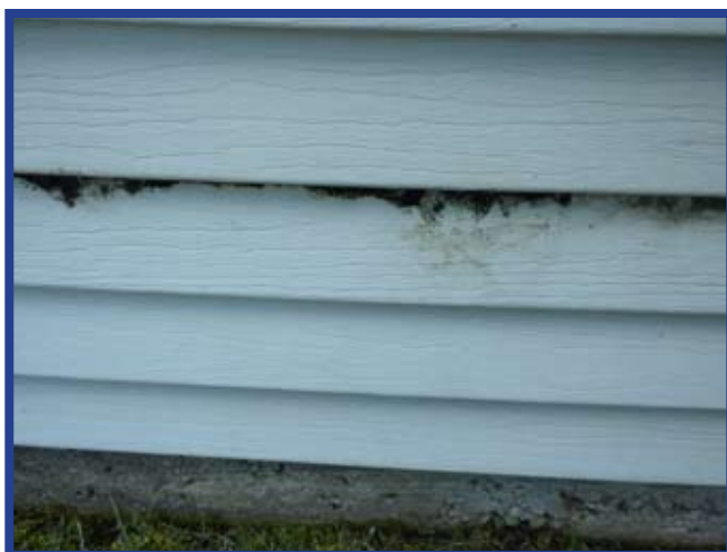
Closeup - Siding - mold under lap boards - Before
