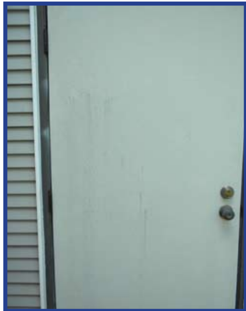
Closeup - Mildew on door backside - Before
